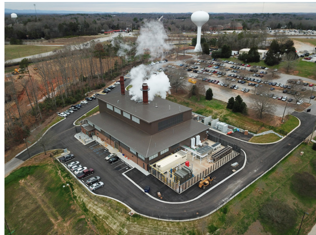
Figure 6. The Duke Energy CHP system at Clemson University in South Carolina. Source: Duke Energy
